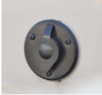
Exterior Cable TV Connection (Located near entrance door) -Typical View
