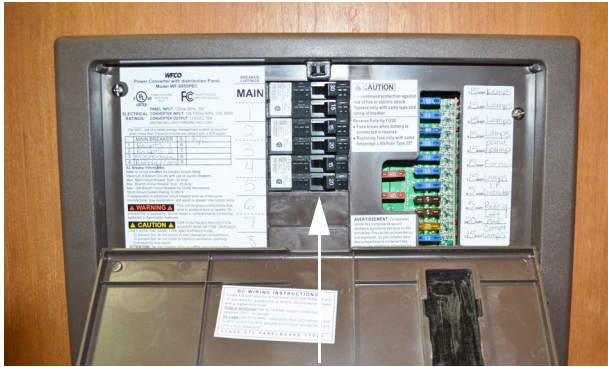
120-Volt Circuit Breakers -Typical View
